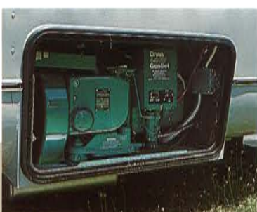
ONAN 110V, 4000W generator.
