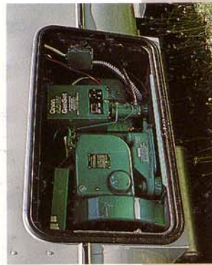
ONAN 110V, 4000W generator.
