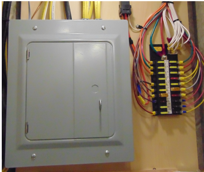
Class A House Fuse Panel Example
