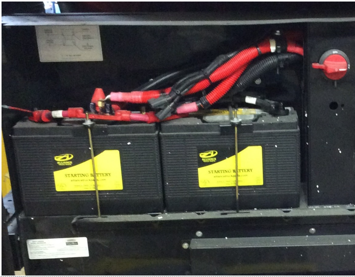
Chassis Battery Bank Example
