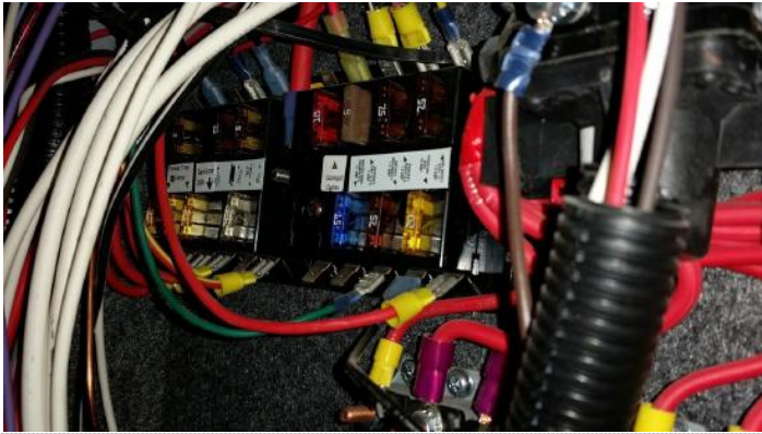
Sample: Cord Compartment Mini-Breakers
