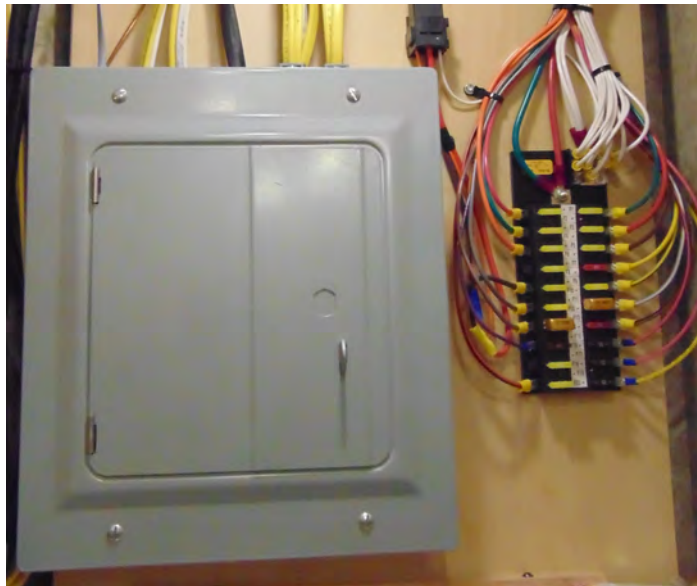
Class A House Fuse Panel Example
