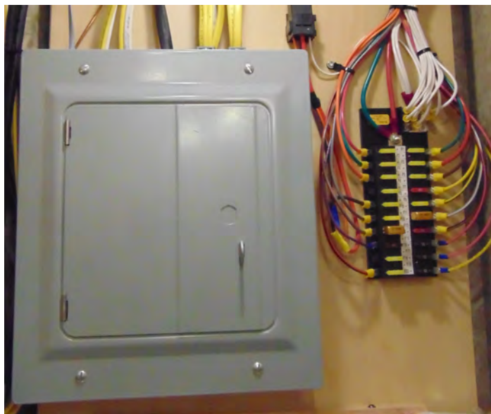
Class A House Fuse Panel Example
