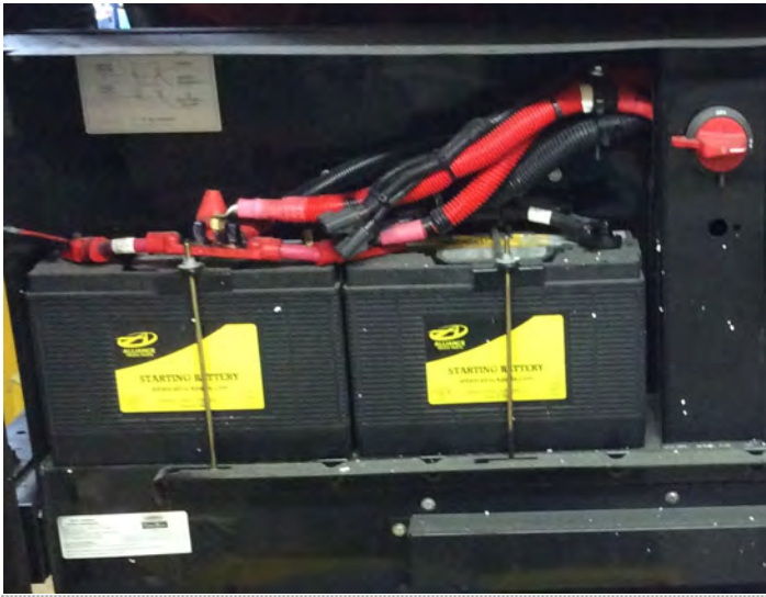
Chassis Battery Bank Example
