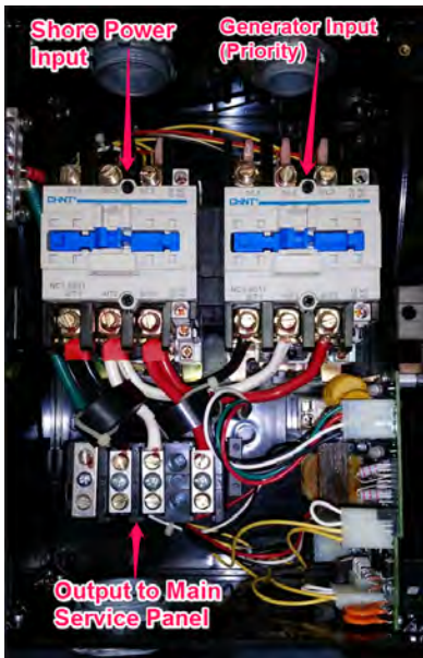
Interior view of a Transfer Switch
