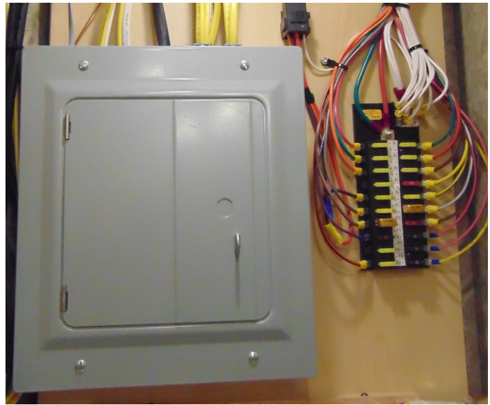
Class A House Fuse Panel Example
