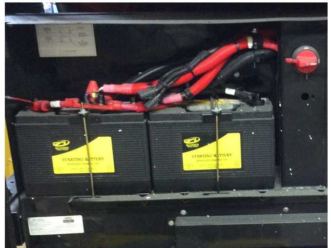
Chassis Battery Bank Example
