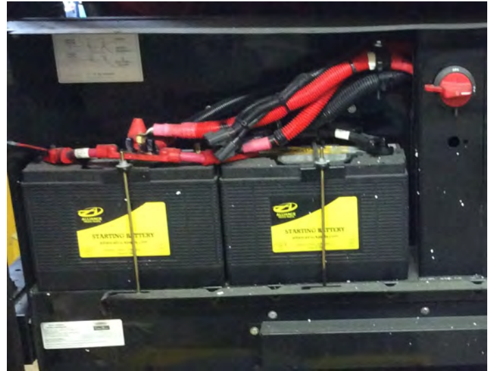
Chassis Battery Bank Example
