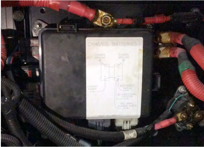
Freightliner Chassis Fuse Panel Example
