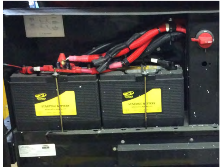
Chassis Battery Bank Example
