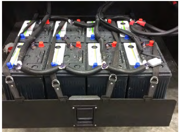
House Battery Bank Example
