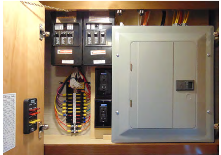
Diesel Pusher Fuse Panel Example
