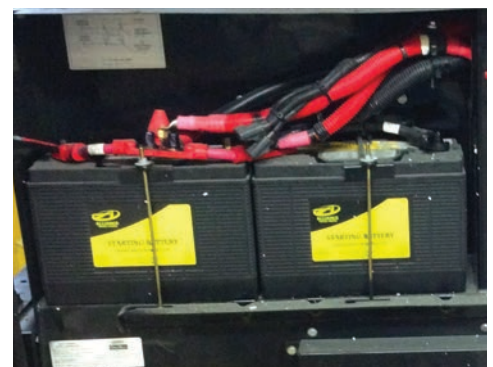
Chassis Battery Bank Example
