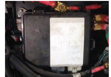
Freightliner Chassis Fuse Panel Example
