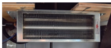
Oasis Basement Heat Exchanger
