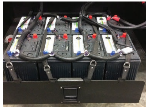
House Battery Bank Example
