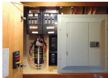
Diesel Pusher Fuse Panel Example
