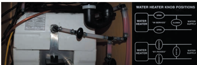
3 Bypass Valve System
