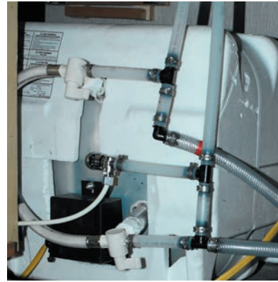
2 Bypass Valve System
