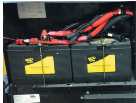
Chassis Battery Bank Example
