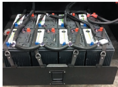
House Battery Bank Example
