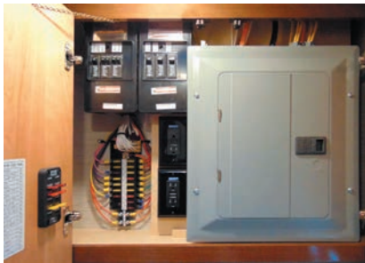
Diesel Pusher Fuse Panel Example
