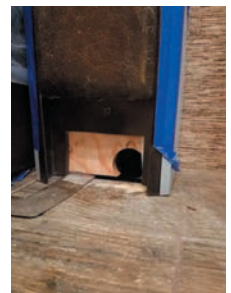
King Aire Access Point
