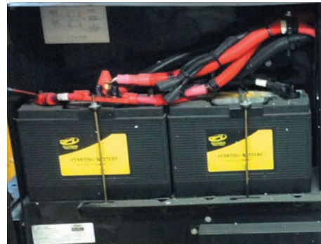
Chassis Battery Bank Example
