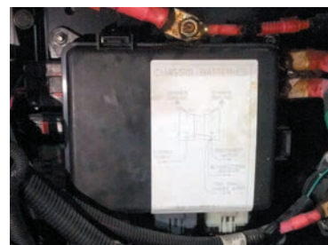
Freightliner Chassis Fuse Panel Example
