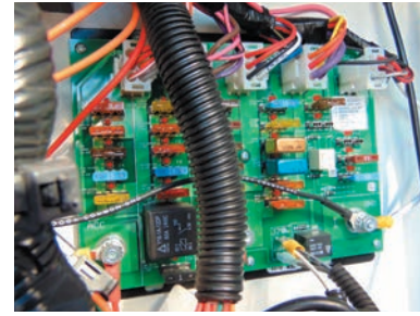
Example of a KIB Fuse Panel
