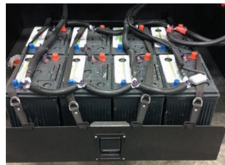
House Battery Bank Example
