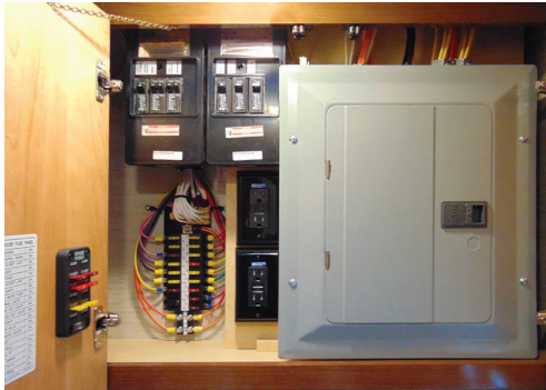
Diesel Pusher Fuse Panel Example
