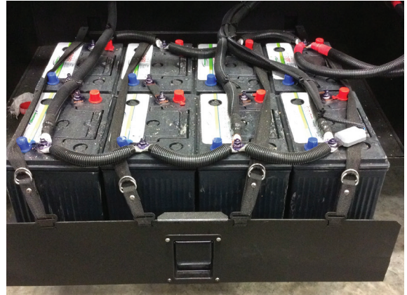
House Battery Bank Example
