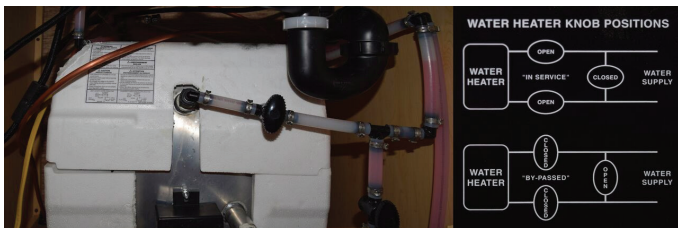
3 Bypass Valve System
