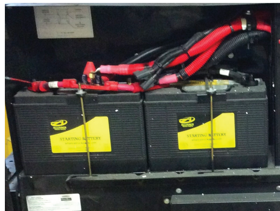
Chassis Battery Bank Example
