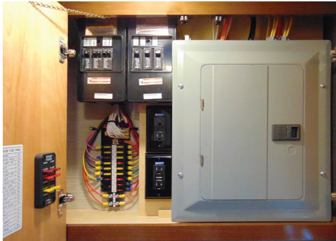
Diesel Pusher Fuse Panel Example
