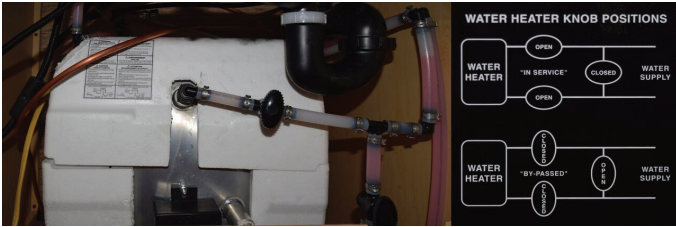
3 Bypass Valve System
