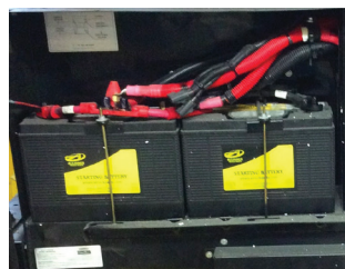
Chassis Battery Bank Example
