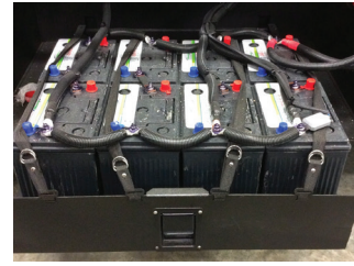
AMG House Battery Bank Example
